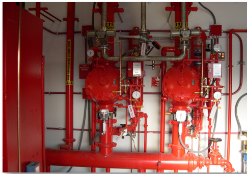
Grunau installed new fire protection equipment at the military base
