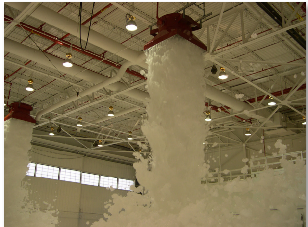
Testing the newly installed high expansion foam system
